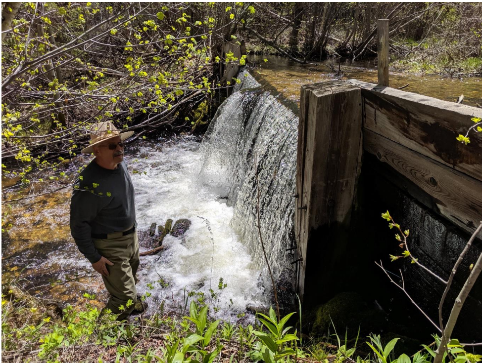
FIGURE 2. PHOTOGRAPH OF BLACK HOLLOW FISH BARRIER DEPICTING CONDITION OF TIMBERS AND LOCAL BANK STABILITY FROM 2019 (FROM USDA FOREST SERVICE 2019).
